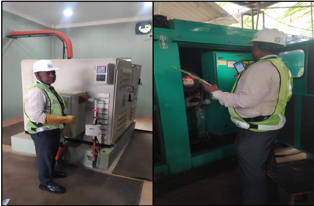
Energy conservation facilities observed in the Campus
